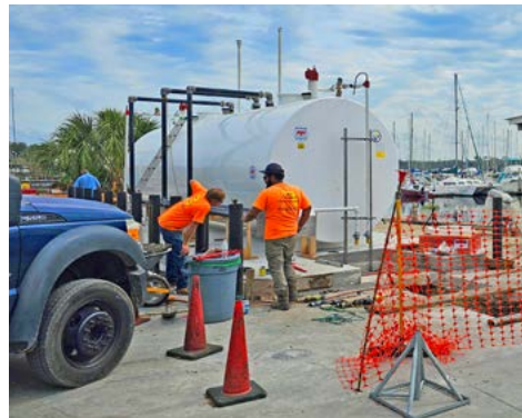
Crews working to install the new fuel tanks Windward Marina Group has brought to the marina.
