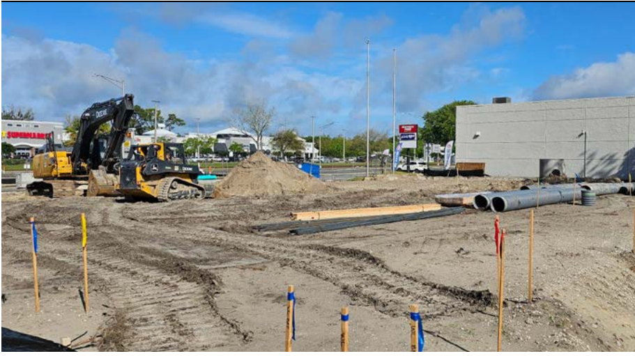
Construction is underway for a proposed shopping center and parking lot expansion along Roosevelt Boulevard in the Fairfax area.
